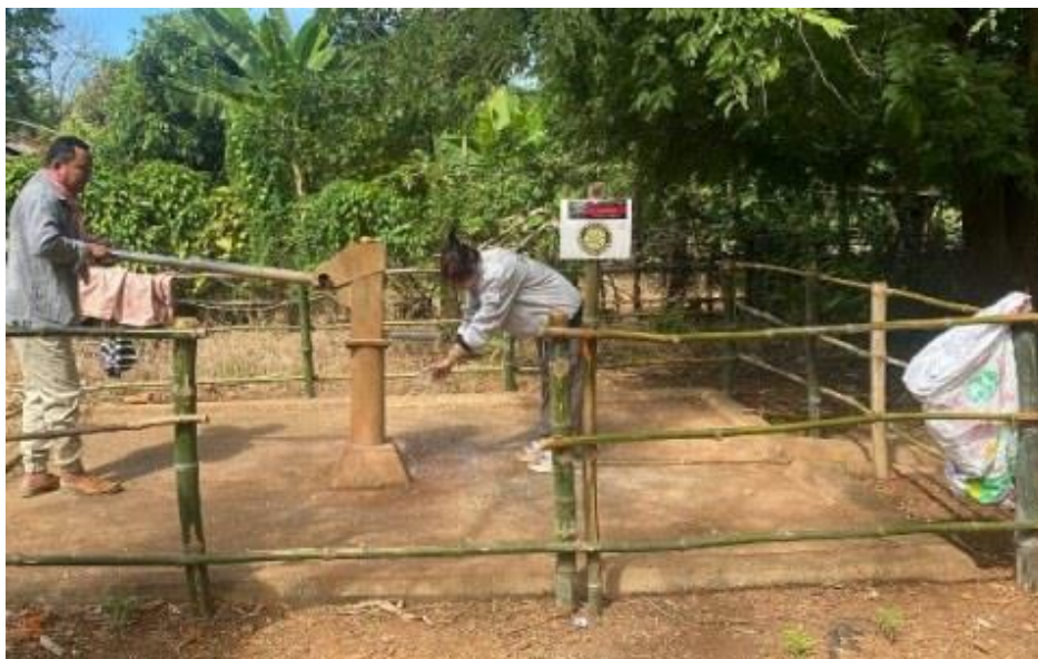
We finally fixed it, this pump well is using by community families;
